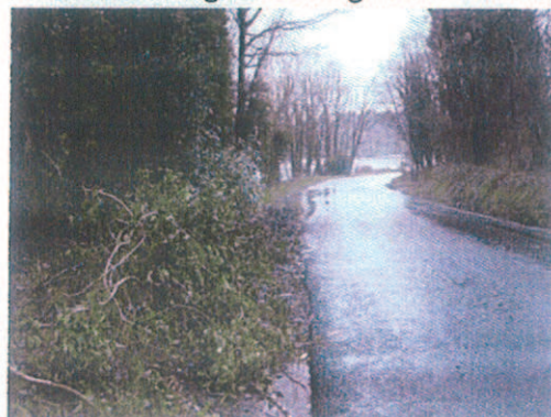
6. Verge blocked looking South
