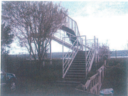
Footbridge over the Railway line at the south west end of Ferry Road.
