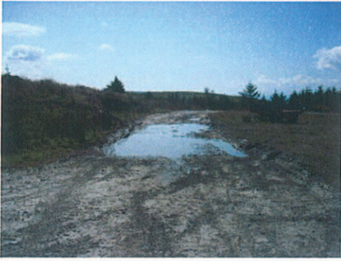
Area of pooling on track
