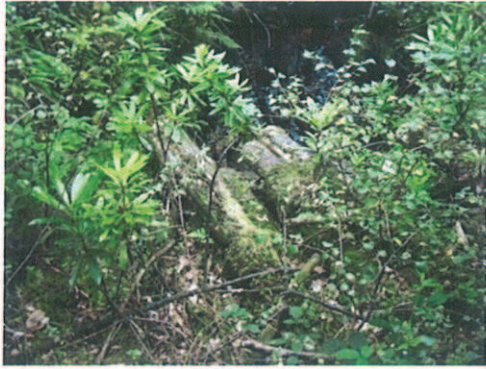
Old bridge that is overgrown and appears to be in a poor condition however it is not known if it is structurally sound
