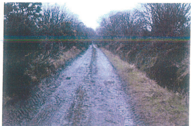
The track through the golf course is generally in a good condition
