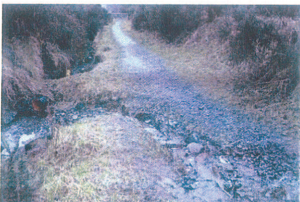
Although there are sections that have suffered from erosion
